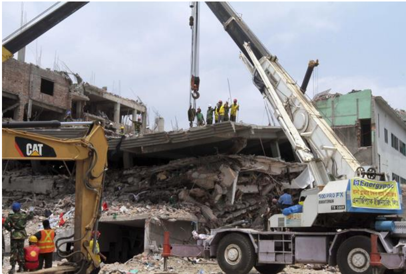
The collapsed Rana Plaza in Bangladesh.
